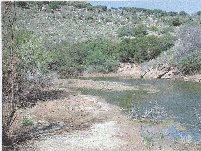
Figure 19. View from dam wall showing sediment laden impoundment.
