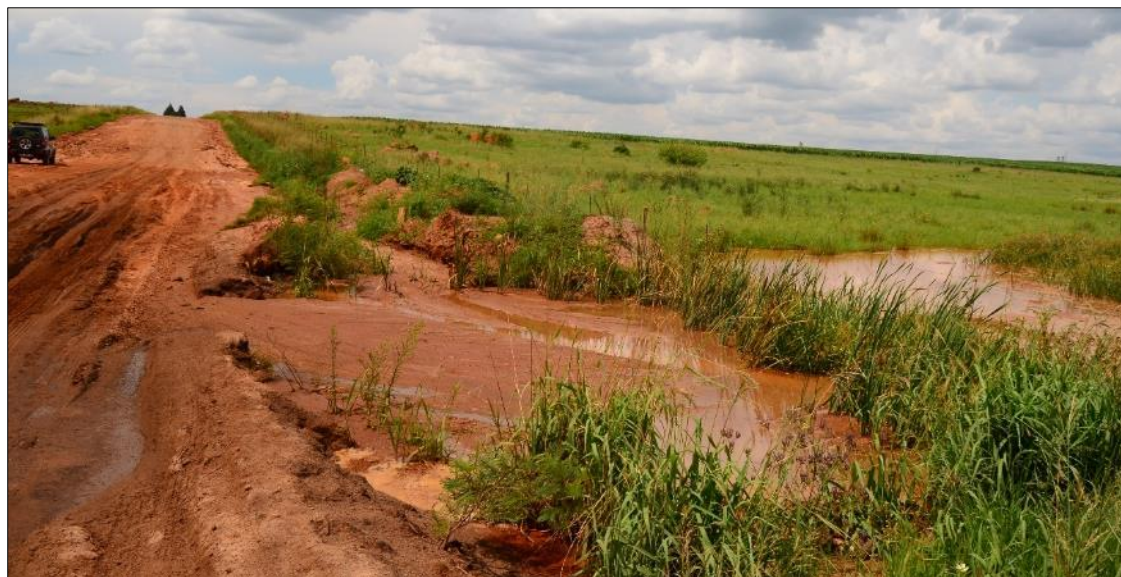
Figure 8: Heavy sedimentation and smothering of instream channel from poorly maintained dirt road
