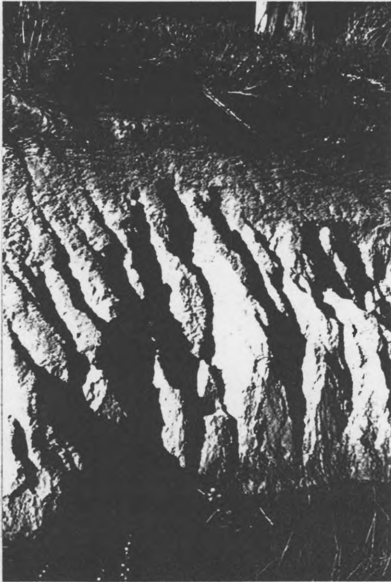
Plates 4. & 5. Canal bank erosion.
