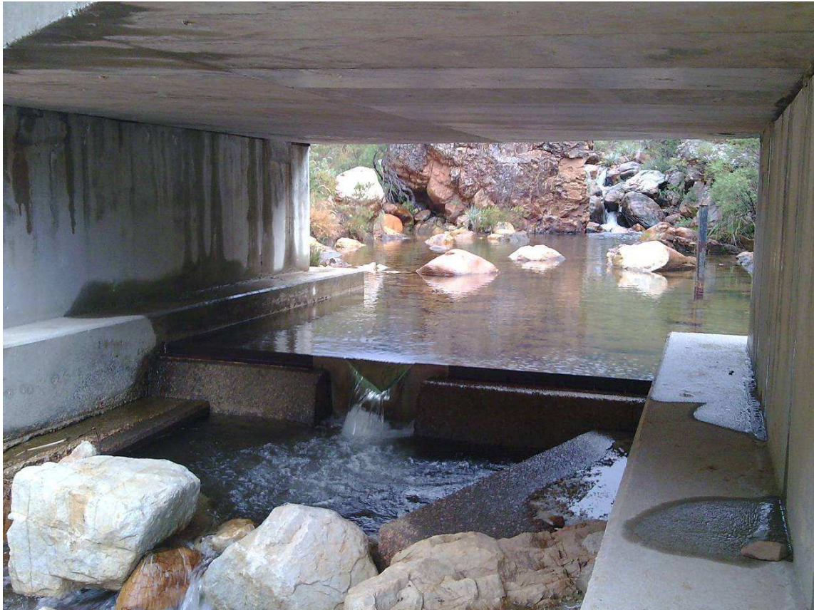
Figure 5-1: Weir 3 on the Koekedouw River
